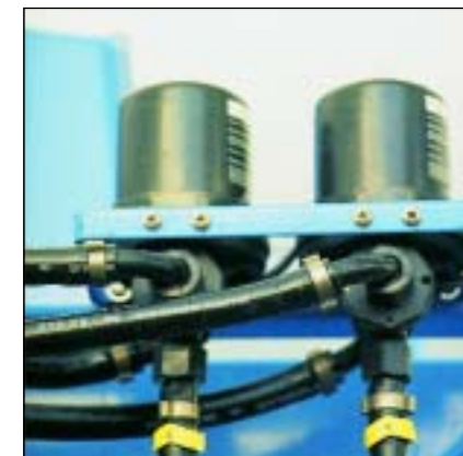
7 - 1/4 turn stainless steel motorised ball valves to resist inclement weather and the various chemical products applied, including, specifically, liquid fertilisers.
